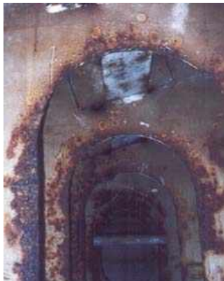
Fig. 5 Corrosion in Ballast Tanks
